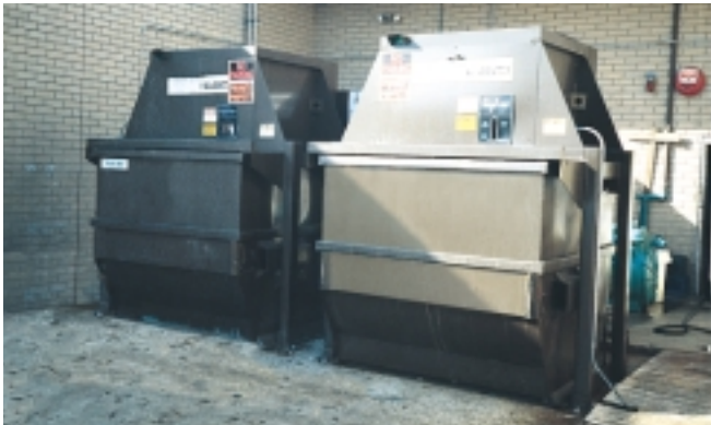
Five 8 yard VIP's, three for corrugated and two for waste, are installed at a shopping mall in Alamance County, NC. These VIP's also reduce the number of hauls through compaction, are conveniently located for mall tenants, and eliminate contamination of recyclables.
